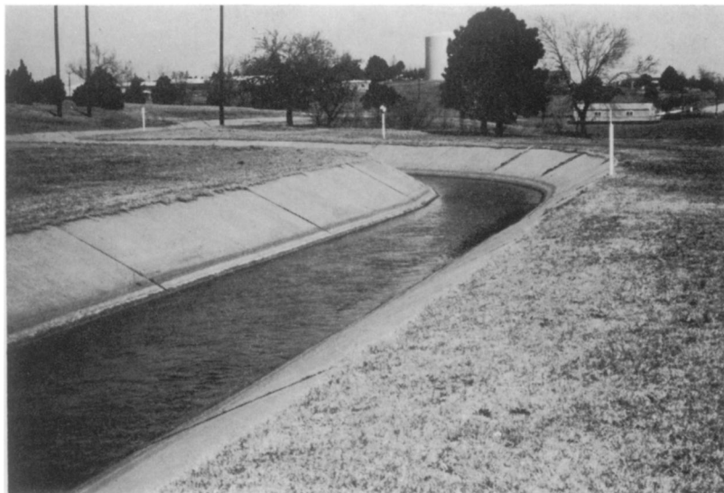
FIG. 1. Canal for transporting heated water to the lake.
